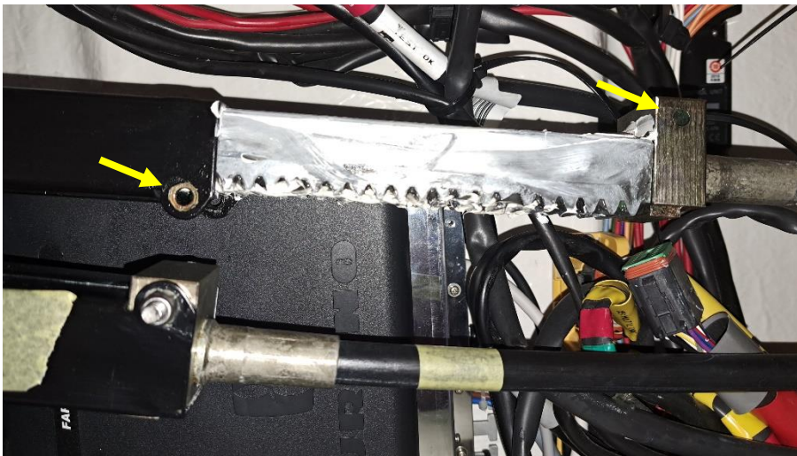
Pic 9: The front rack is in position. The second is on it's way – BUT: the brass stopper is mounted 180° wrong. In this case the bore has to be on the lower side to meet the holes at the end of the housing.
